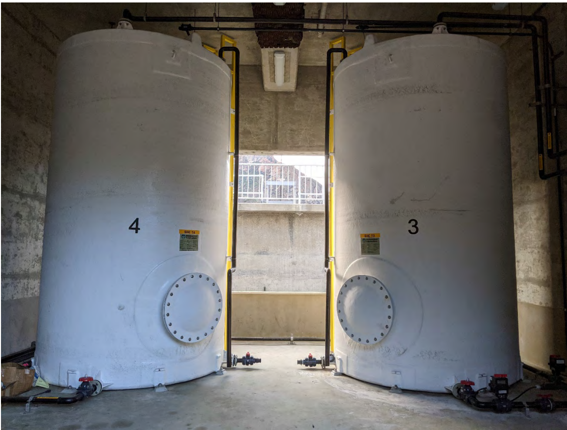
Figure 2: Upper Chemical Room Tanks 3 and 4
